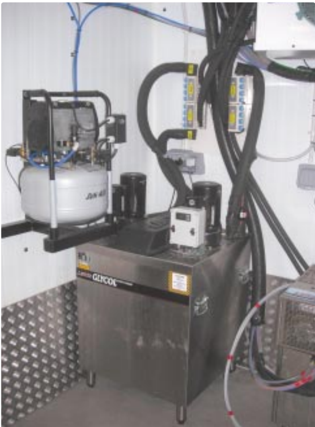
The large glycol cooler and compressor which is central to City Dispense Services' 'Pub of the Future'.
