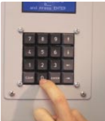
Figure 7: Cellar control panel of an automated cleaning system using a digital display. – Photo supplied by BLCS Ltd
